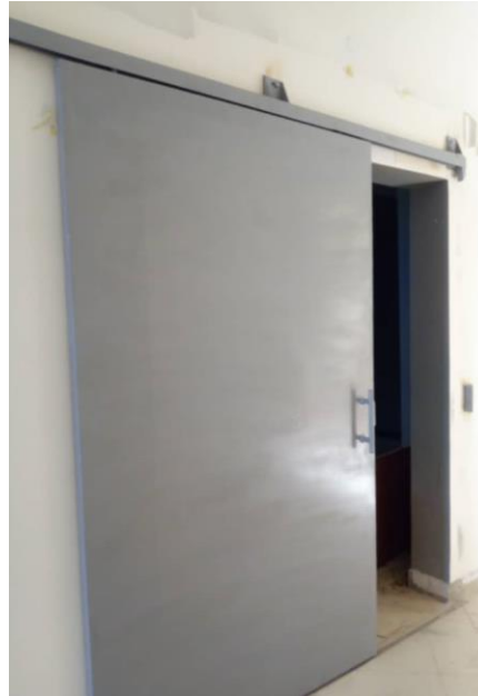
TEMDO radiation protection Doors installed at Bariadi Referral Hospital X-Rays and ICT scan laboratories.
